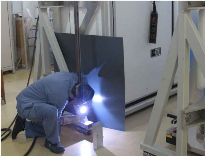
FIG. 15.8 – Welding work for reinforcement of the transportation frame done directly on a FlashCam camera body.
