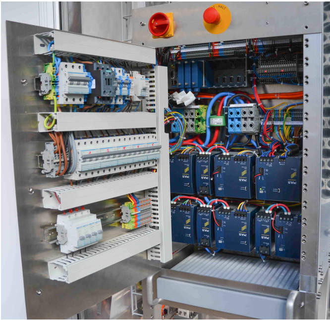
FIG. 6.5 – The safety control cabinet with circuit breakers for the 230 VAC safety and 3x400 VAC physics power and the redundant 24 VDC power supplies. The cRIO control system is installed at the top left side.
